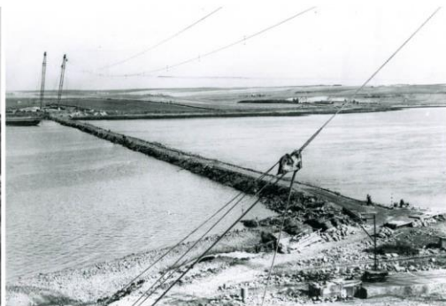
August 1943. The barrier nearing completion as seen from Lamb Holm. Note the aerial ropeways.
